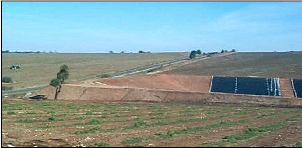
Plaque 1: An irrigation storage in the Clare Valley showing the prepared soil surface. A geotextile underlay is often used where the soil contains sharp rubble, but in this example, there is none.
