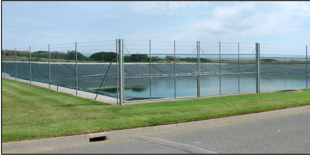
Plaque 5: The treated effluent storage at Christies Beach WWTP. Note the varying freeboard – instead of cutting a bench at a fixed elevation, the liner was continued up the slope to the left until it was convenient to return it into the ground.
