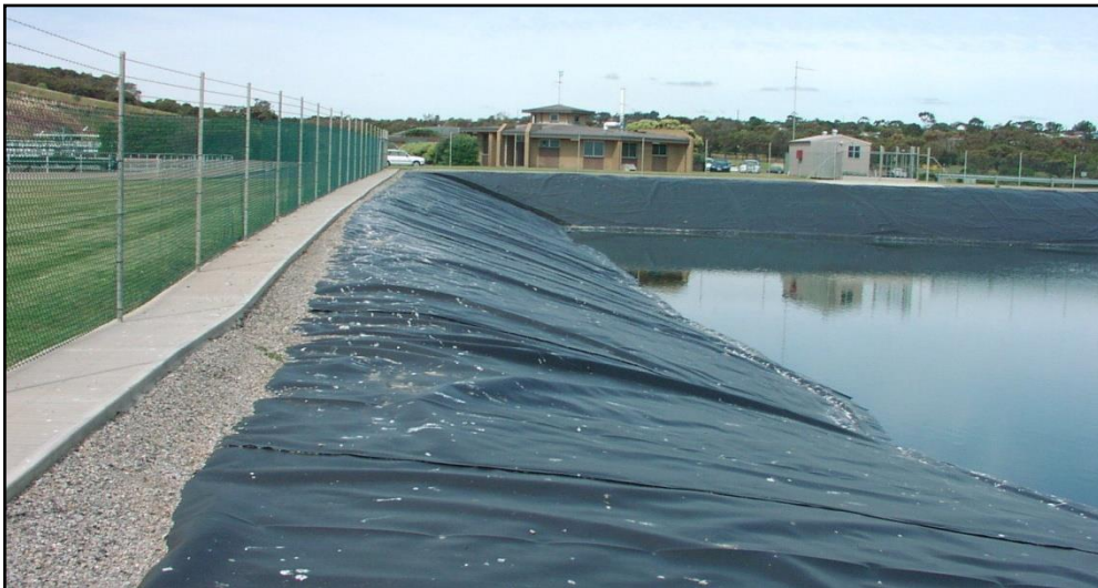
Plaque 6: The treated effluent storage at Christies Beach WWTP. The fence has a concrete footing/path and the liner is simply returned into a backfilled trench. It is required to avoid having sharp aggregates anywhere near a liner.
