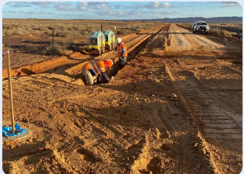
Workers from Aboriginal-owned recruitment service, RAW, replaced 22.5km of pipeline between Copley and Lyndhurst.
