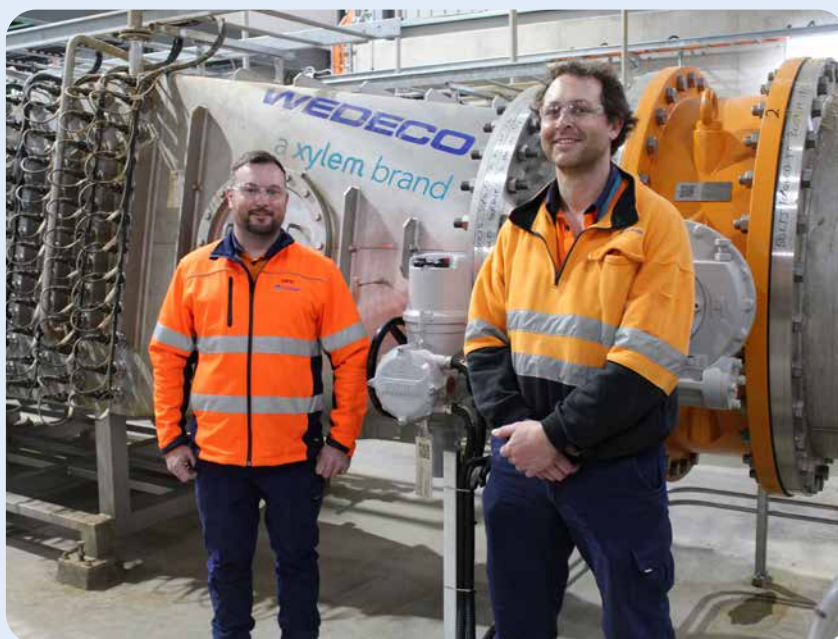
Project Coordinator David Flaherty and Plant Supervisor Ian Holmes at Happy Valley Water Treatment Plant with UV disinfection reactor.
