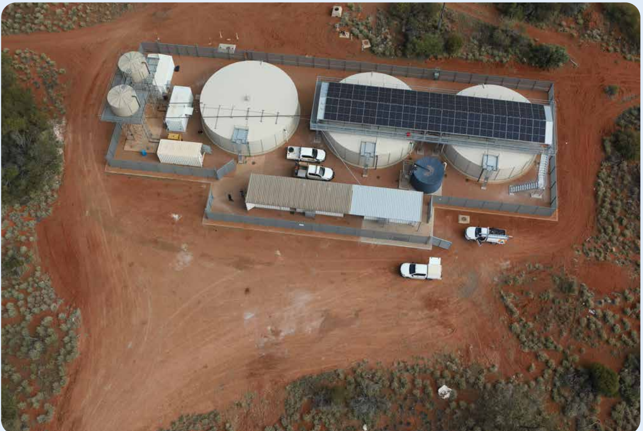
Kaltjiti Desalination Plant with solar panels.
